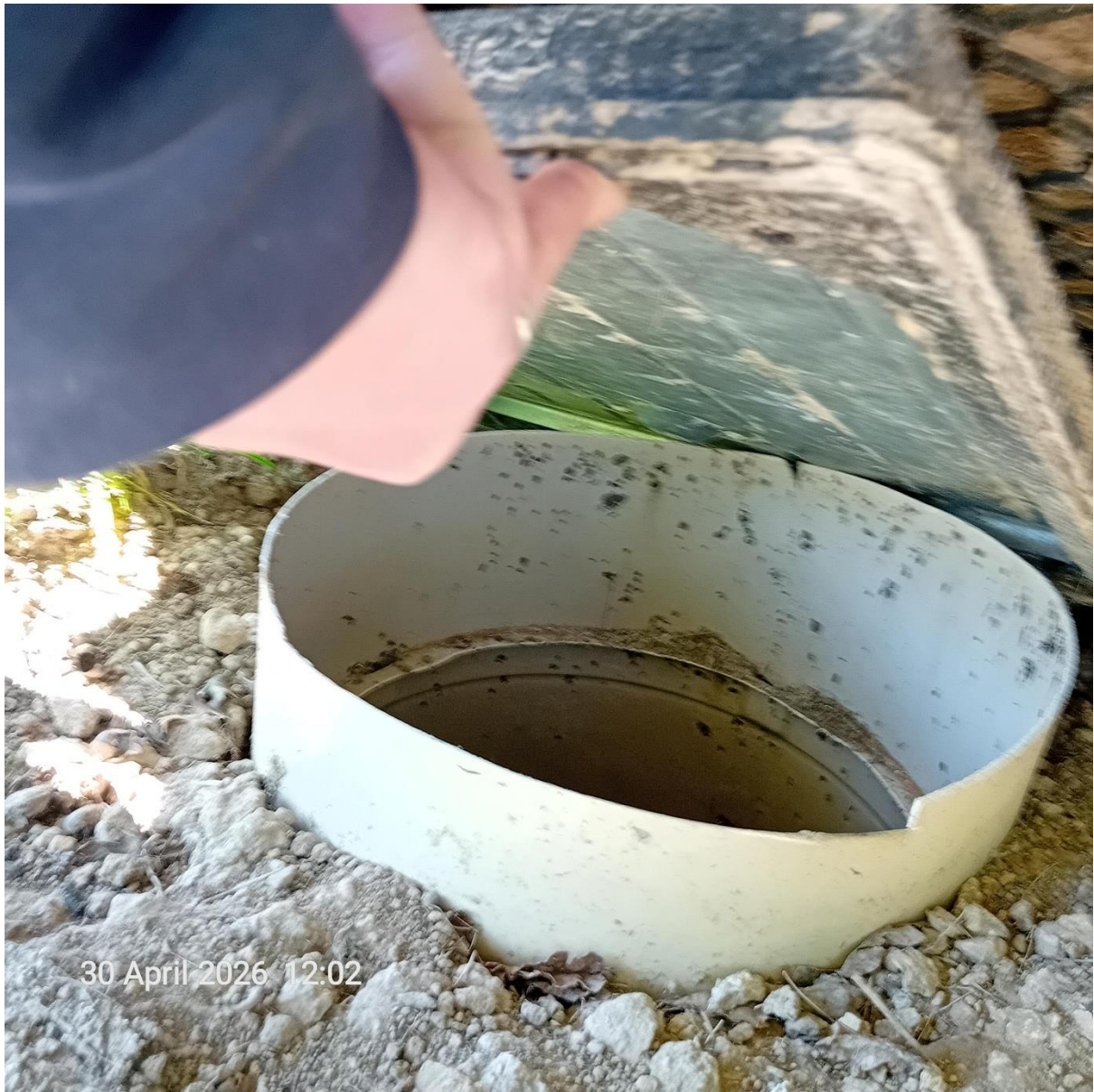
AC164 Photograph of plot 4 showing the opening to the large foul water treatment plant which had been concealed.
