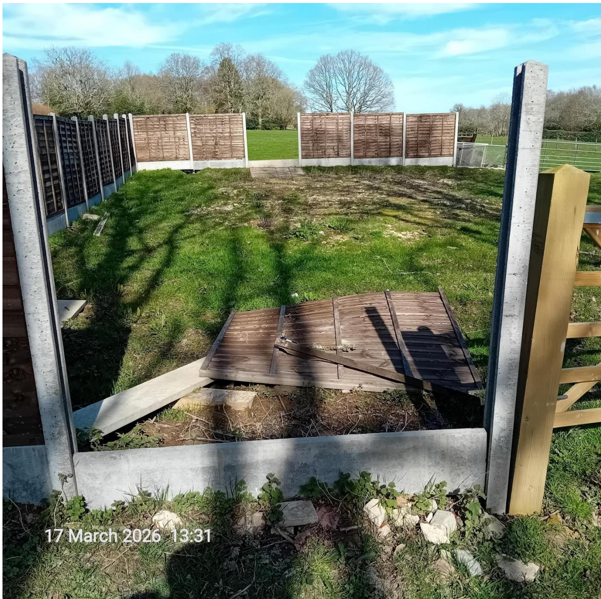
AC146 photograph of plot 2 showing damaged fence panels.
